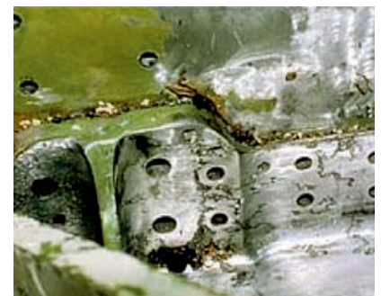
Figure 2 Example of pitting corrosion
