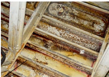
Figure 8 Accumulation of corrosive "products" below a leaking toilet could reduce the thickness of the structure (hence the strength). Aside from the potential health concerns, this may lead to structural failure (decompression)
